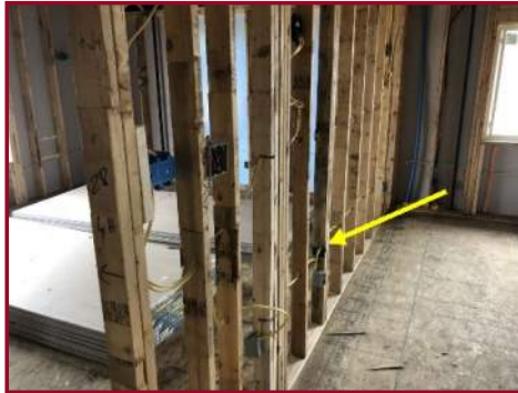
PROTECTIVE WIRING PLATES NEEDED IN DINING ROOM
