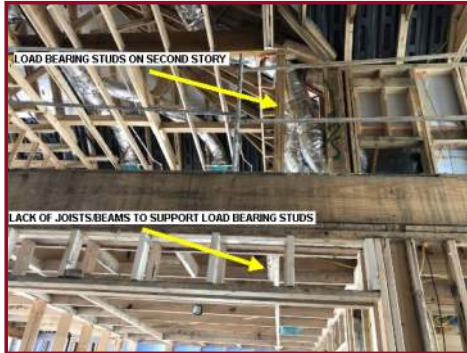
LACK OF PROPER BEAM SUPPORT FOR LOAD BEARING STUDS
