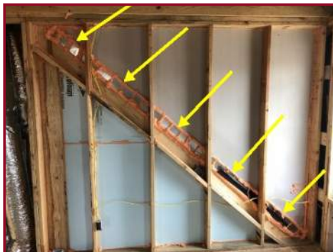
IMPROPER FLASHING INSTALLATION
