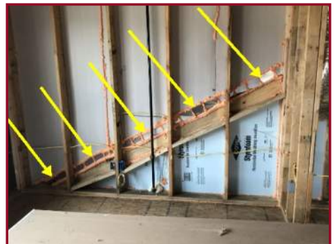
IMPROPER FLASHING INSTALLATION
