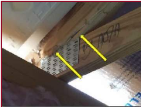
DAMAGED TOP CHORD TO TRUSS
