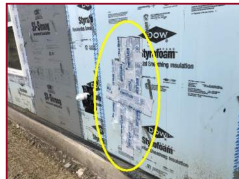
EXTERIOR SHEATHING DAMAGE ON NORTH SIDE
