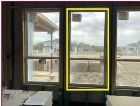
WINDOW OUT OF SQUARE WITH OPENING
