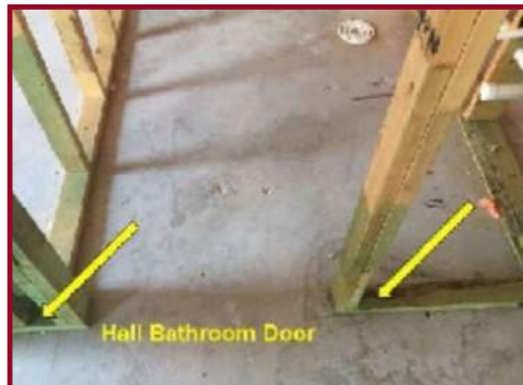
SILL PLATES NEED TO BE SECURED ON BOTH SIDES OF DOOR
