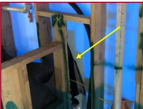
EXTERIOR SHEATHING DAMAGE ON NORTH SIDE OF MASTER BATHROOM
