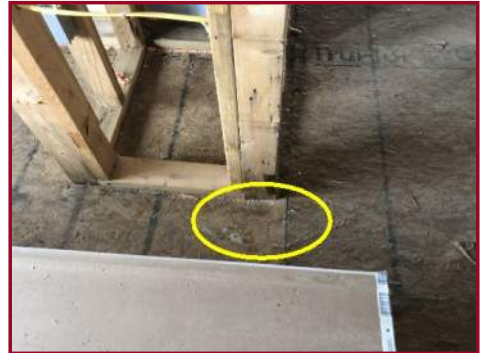
DECKING SAGGING UNDER LOAD BEARING STUDS FROM LACK OF SUPPORT BEAMS BELOW
