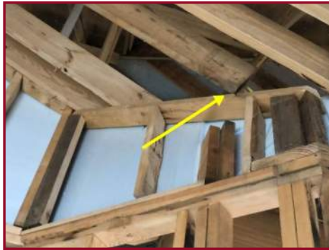
JOIST IS TOO SHORT AND DOES NOT HAVE PROPER BEARING
