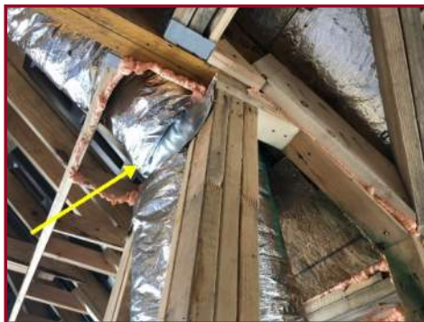
DUCTWORK CRIMPED AT TOP OF STAIRWAY
